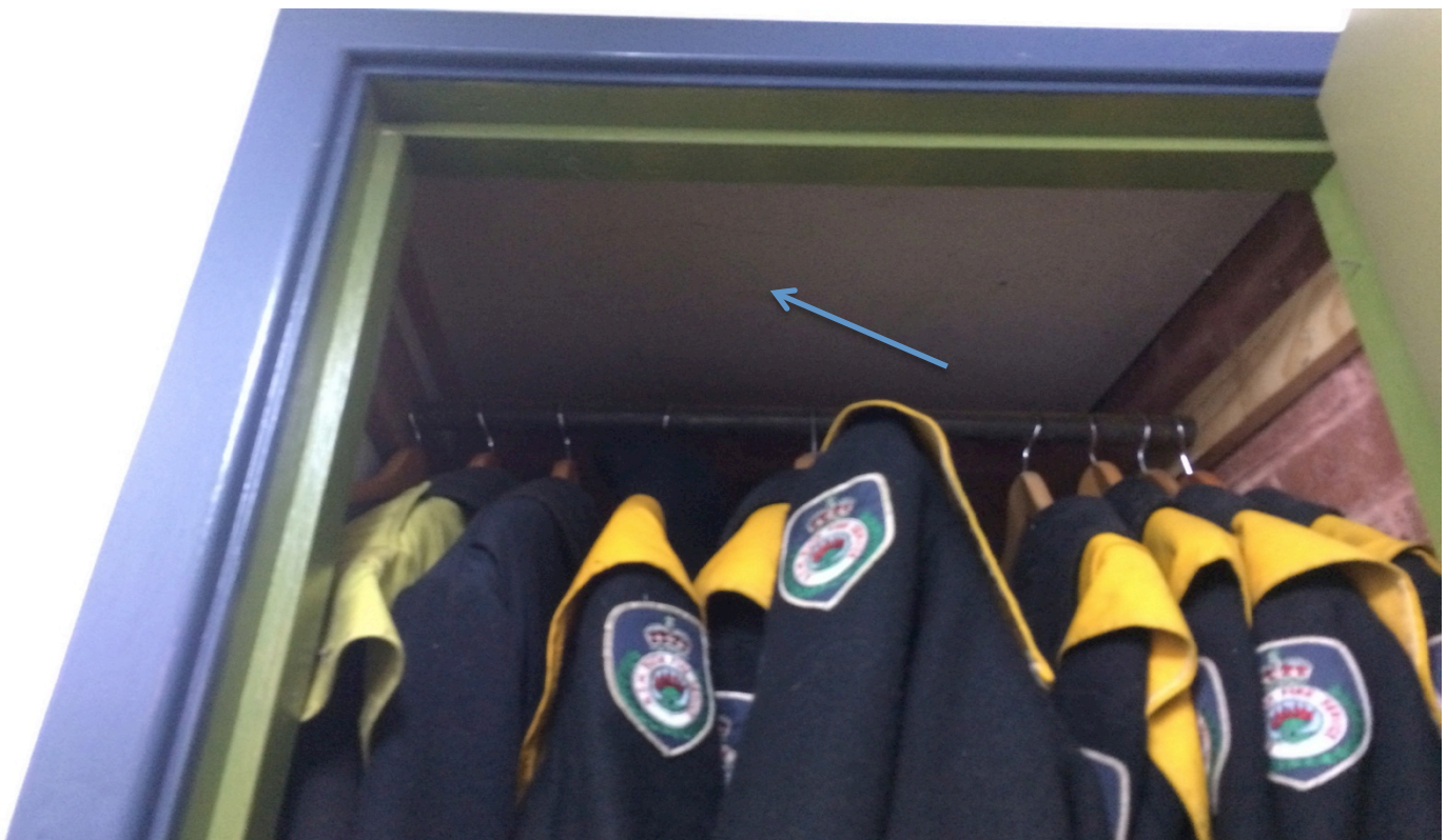
Photo 108: Fibreboard ceiling panel assumed to contain asbestos in the Jacket Storage cupboard in the western garage of the Glenbrook Rural Fire Service Bushfire Station.
