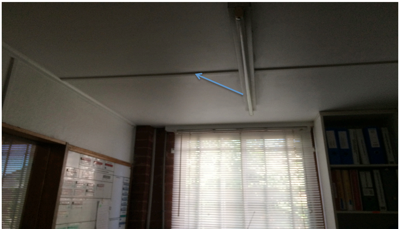
Photo 106: Fibreboard ceiling lining assumed to contain asbestos in the Office in the western garage of the Glenbrook Rural Fire Service Bushfire Station.
