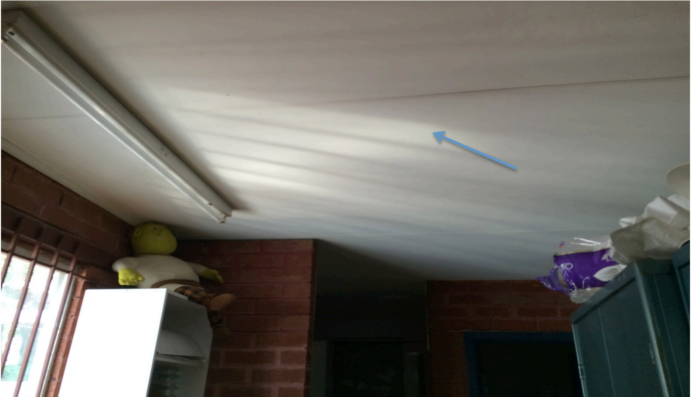
Photo 109: Fibreboard containing asbestos ceiling lining Storage Area and Toilet/Shower area in the western garage of the Glenbrook Rural Fire Service Bushfire Station .
