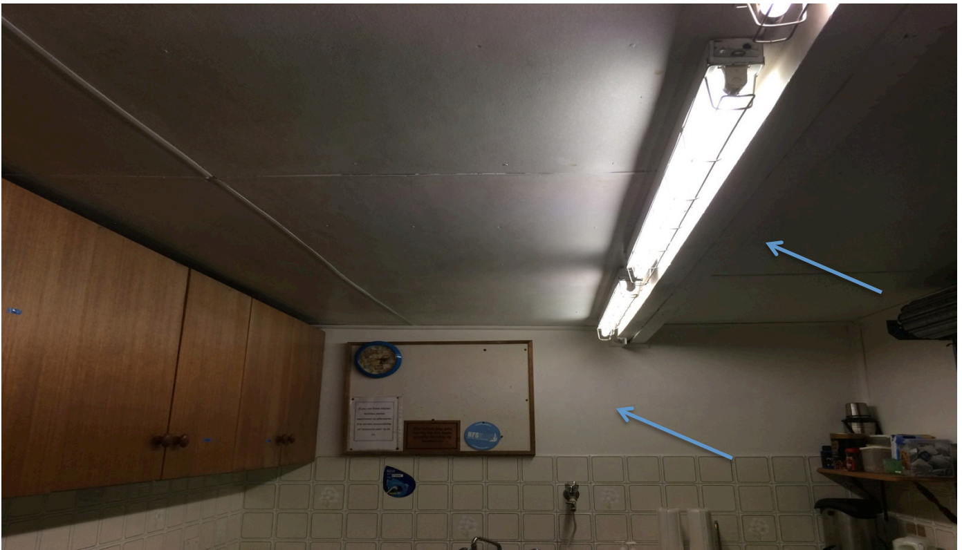
Photo 110: Fibreboard ceiling lining and internal wall cladding assumed to contain asbestos in the Kitchen in the western garage of the Glenbrook Rural Fire Service Bushfire Station .
