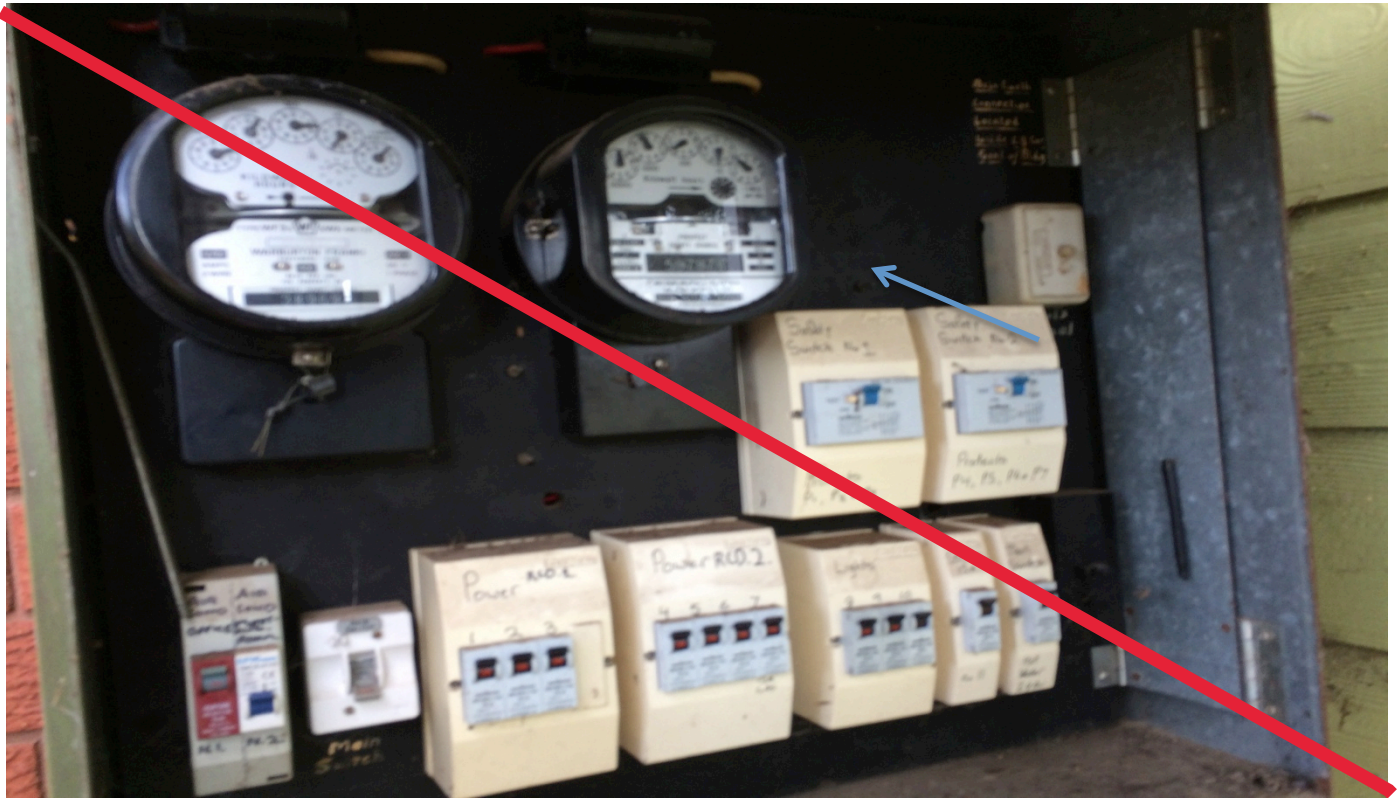
Photo 105: Electrical backing board containing asbestos on the southern perimeter of the Glenbrook Rural Fire Service Bushfire Station.
