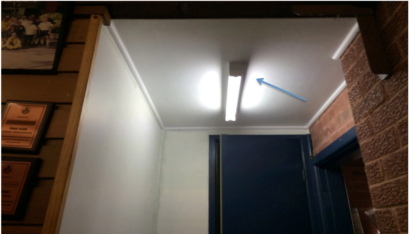
Photo 107: Fibreboard ceiling panel assumed to contain asbestos outside the Jacket Storage cupboard in the western garage of the Glenbrook Rural Fire Service Bushfire Station.
