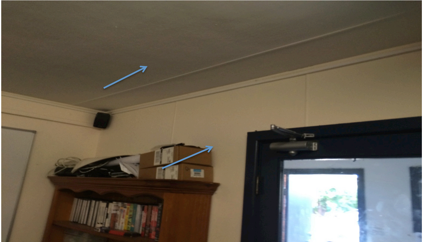
Photo 111: Fibreboard ceiling lining and southern internal wall cladding assumed to contain asbestos in the central meeting room in the western garage of the Glenbrook Rural Fire Service Bushfire Station.
