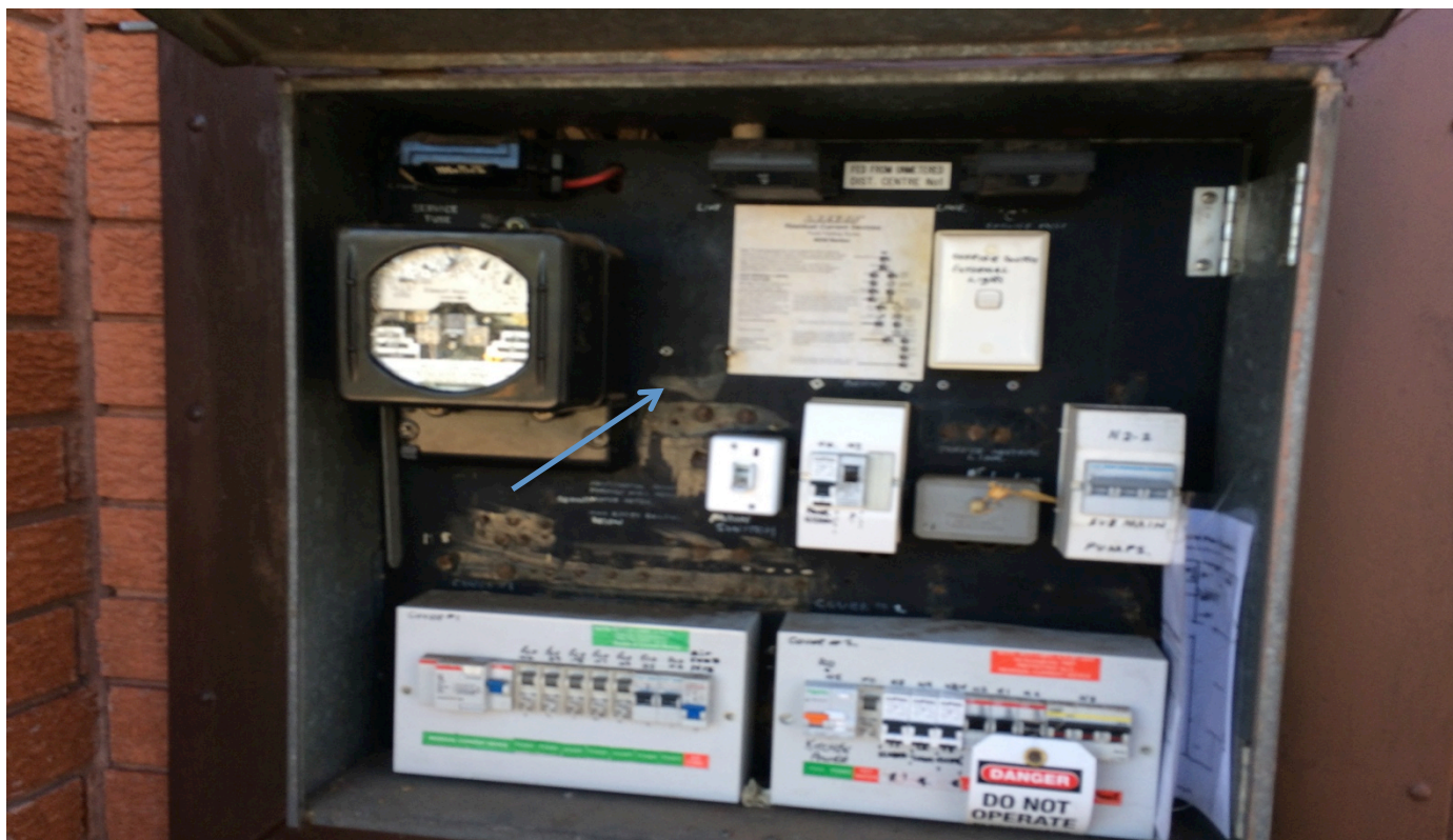
Photo 128: Electrical backing board containing asbestos on the south-western perimeter of the Warrimoo Rural Fire Service Bushfire Brigade.
