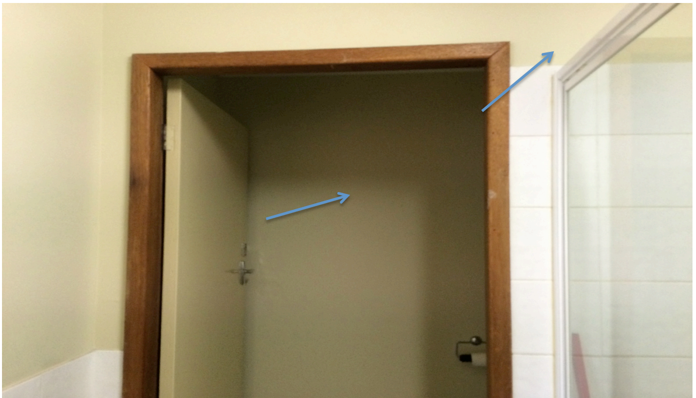
Photo 130: Fibreboard containing asbestos internal wall cladding of the Toilet and Shower in the Warrimoo Rural Fire Service Bushfire Brigade.
