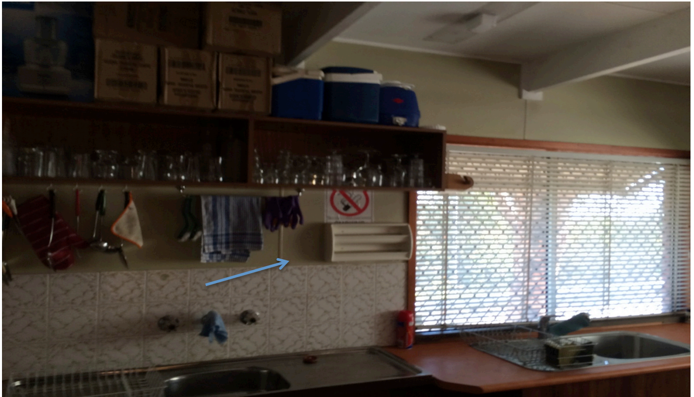
Photo 129: Fibreboard containing asbestos internal wall cladding of the Kitchen in the Warrimoo Rural Fire Service Bushfire Brigade.
